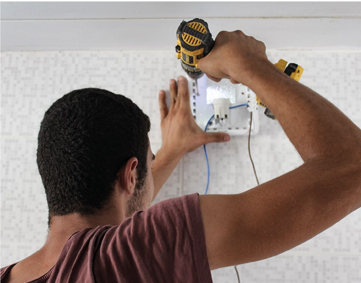
Apprentice Mehmet Göz installing electrical components as part of the Training for Results project.
